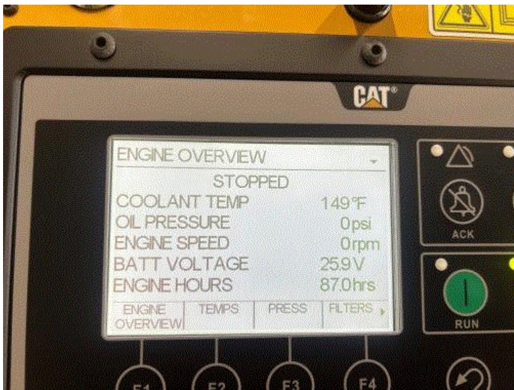
Image 7(Engine control) : EUMERGEN engine control screen showing total engine hours
