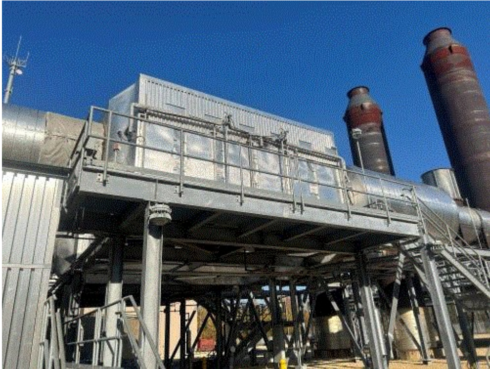
Image 6(SRC control unit) : SRC control unit and stacks
