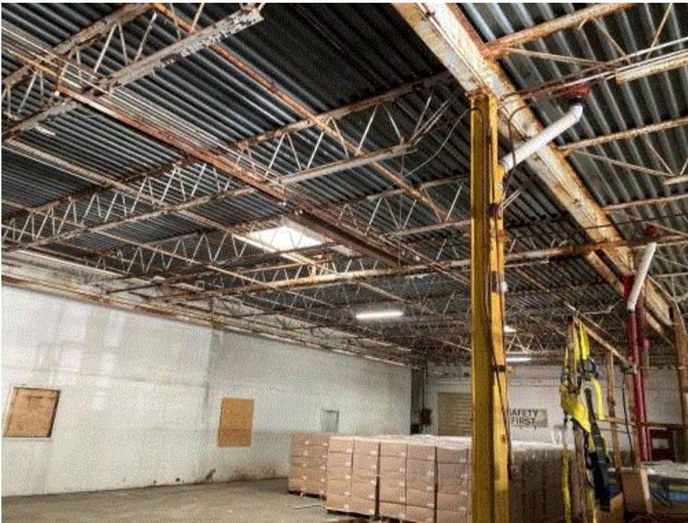
Image 1(Roof 1) : Image of the new roof in the south portion of the facility.
