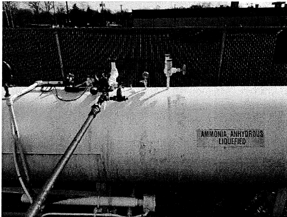
Image 7(Ammonia) : 1000 gallon Ammonia storage tank adjacent to West building.
