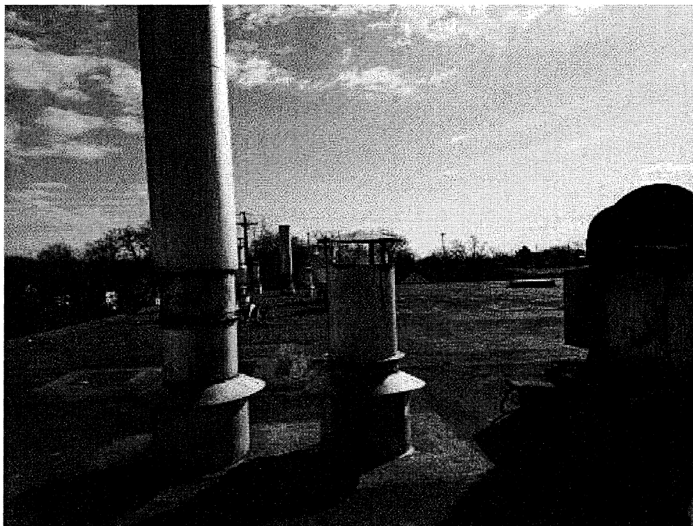
Image 6(Smoke) : Smoke coming from stack with rain cap.
