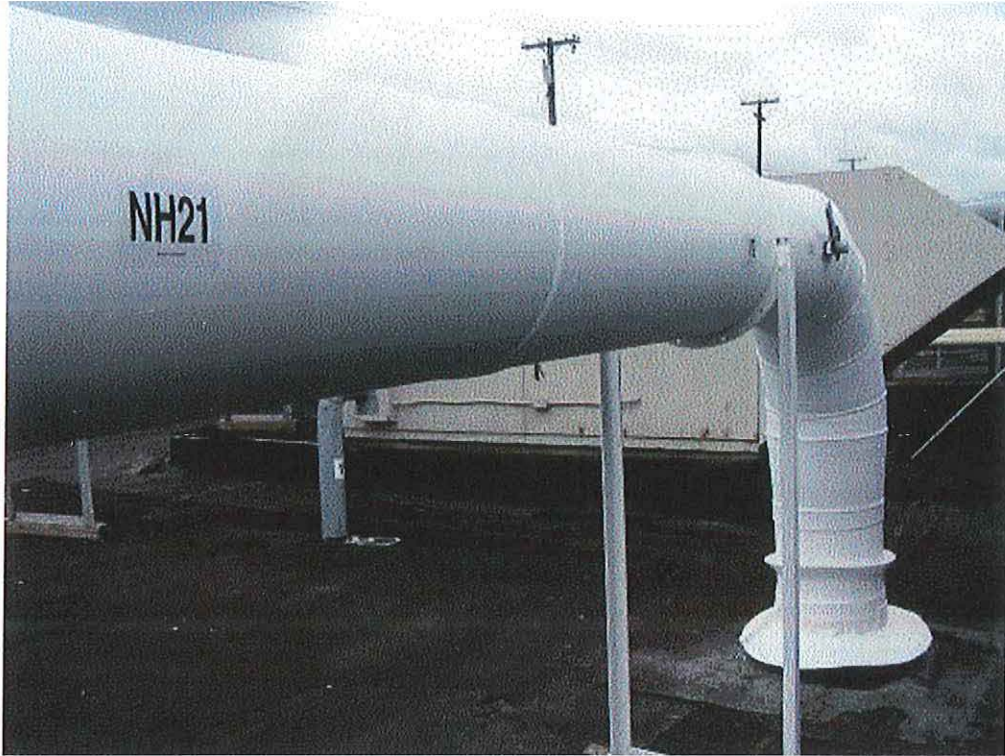
Image 4(4) : Painted ducts with ID Nos.
