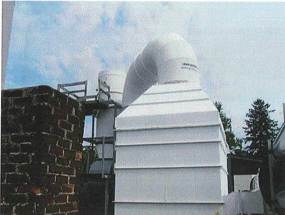
Image 1(1) : South scrubber (No. 3)..
