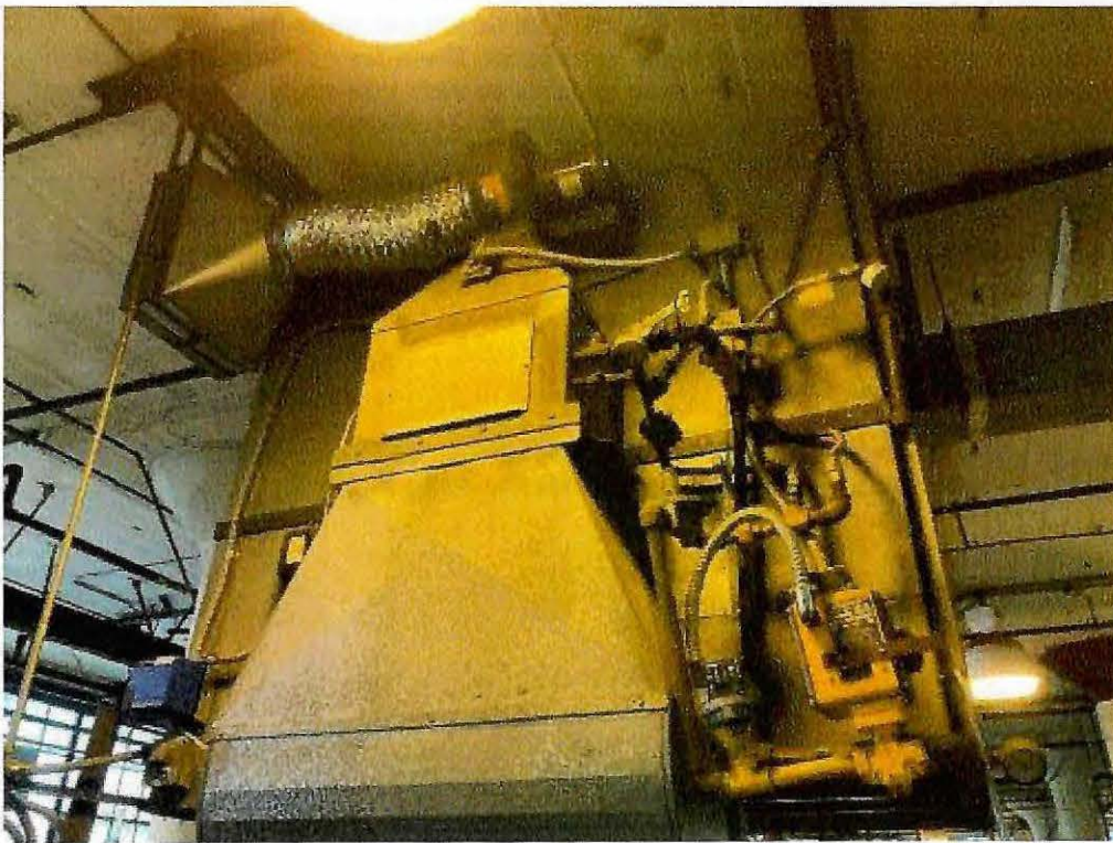
Image 2(Loom Dryer) : Natural gas-fired burner with air intake duct.
