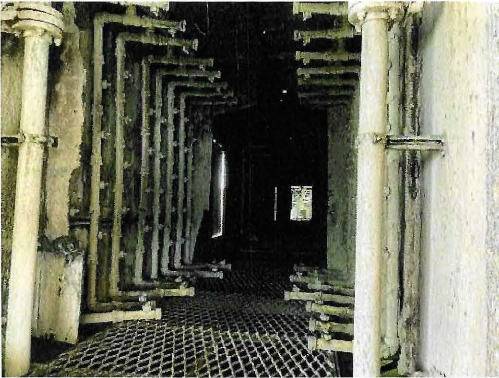
Image 3(Metal Preparation) : Metal surface preparation booth, containing spray nozzles, for frames of furniture.
