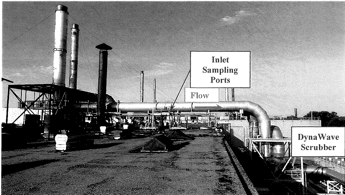
Figure 2-1. No. 1 Biofilter Inlet Sampling Location
