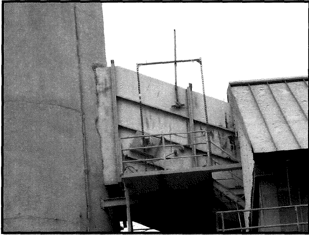
Figure 5-2. Kiln 19 Breeching Duct
