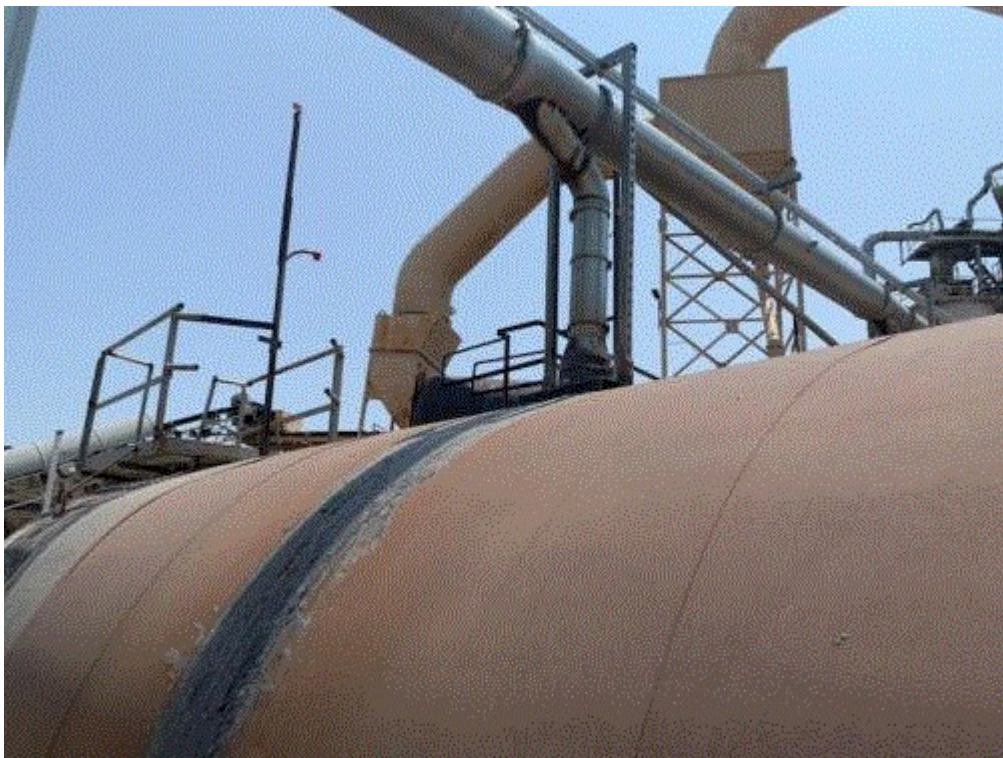
Image 2(Side View AC Tank) : Emissions were noticeable from the area between the pipe and the top of the AC tank. Facility cleaned cartridges and eliminated emissions.
