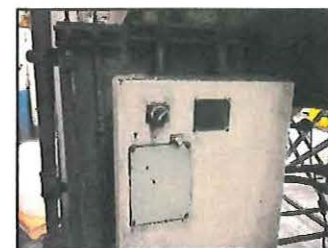
Figure 2 - Elinio Baghouse Pressure Drop display screen. One pressure drop reading related to one baghouse.
