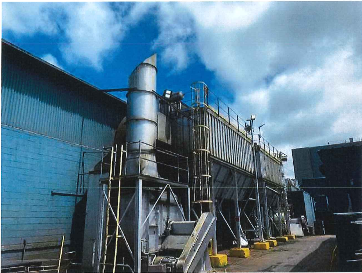
Image (4) West Fuller baghouse stack.
