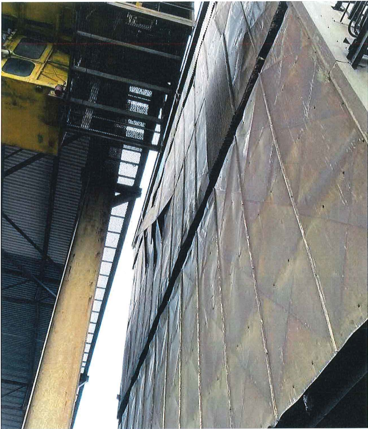
Image (3) Gaps observed in cupola baghouse structure.
