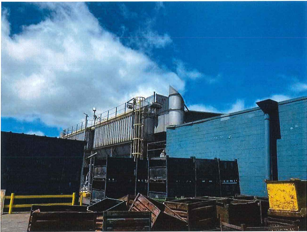
Image (2) East Fuller baghouse stack.
