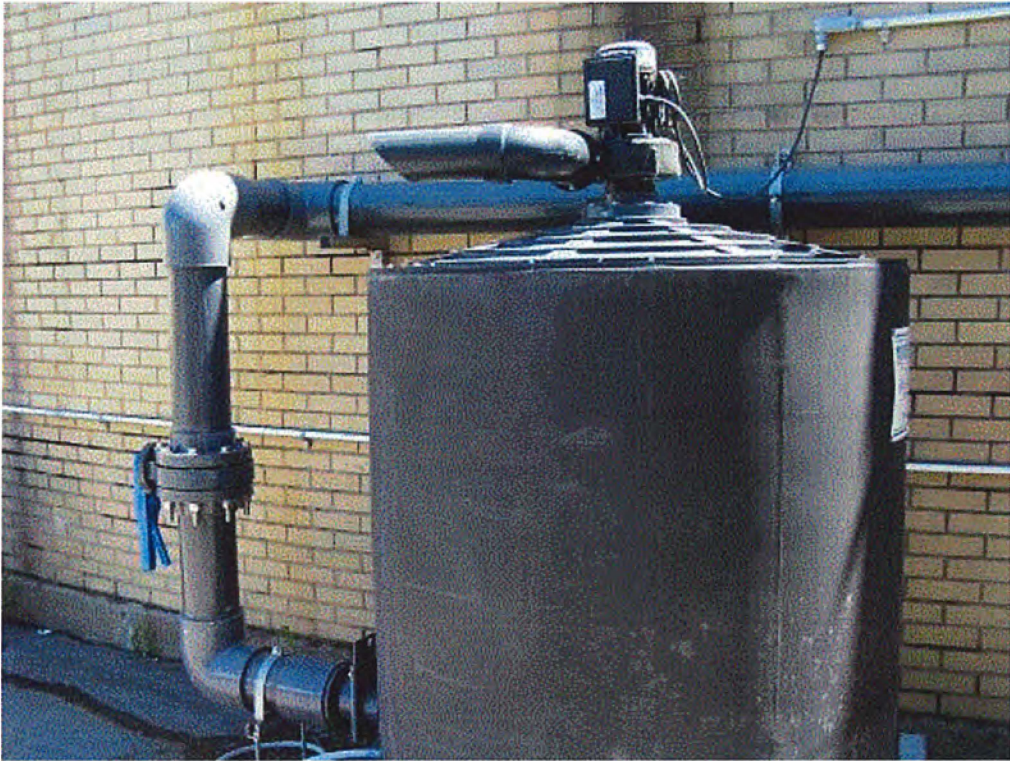
Image 1(001) : 2-stage odor scrubber.
