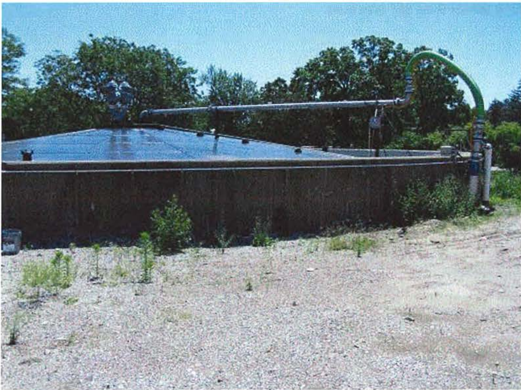
Image 2(002) : South (new) digester.
