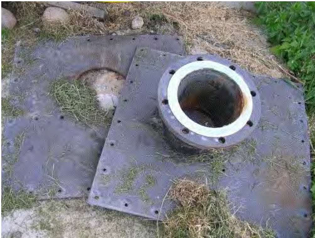
Image 2(002) : Carbon steel plates from digestate tank.
