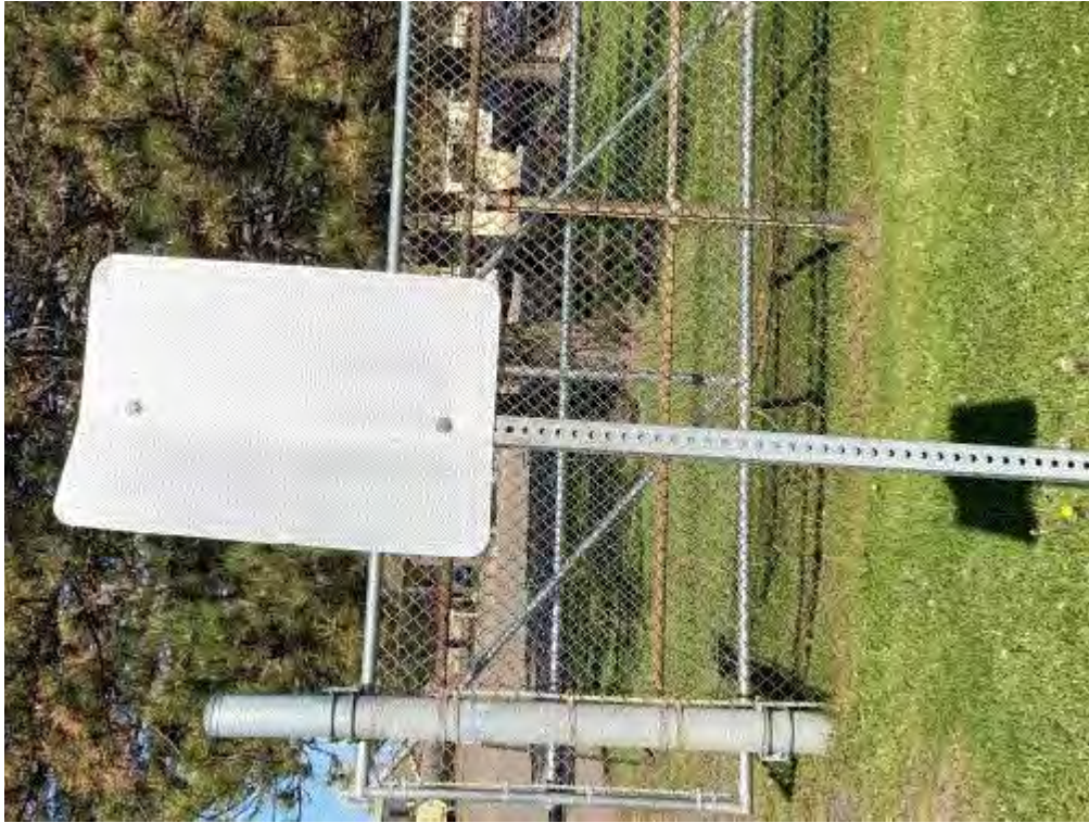
Image 8(Speed Limit sign) : Faded 10 mph speed limit sign during inspection.
