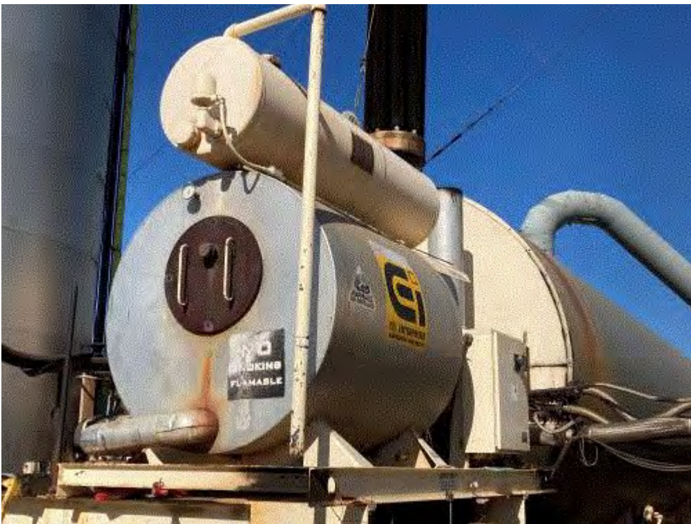
Image 5(Gas-fired boiler) : Natural gas-fired boiler used to heat the heat transfer fluid for warm the AC tanks and silos.
