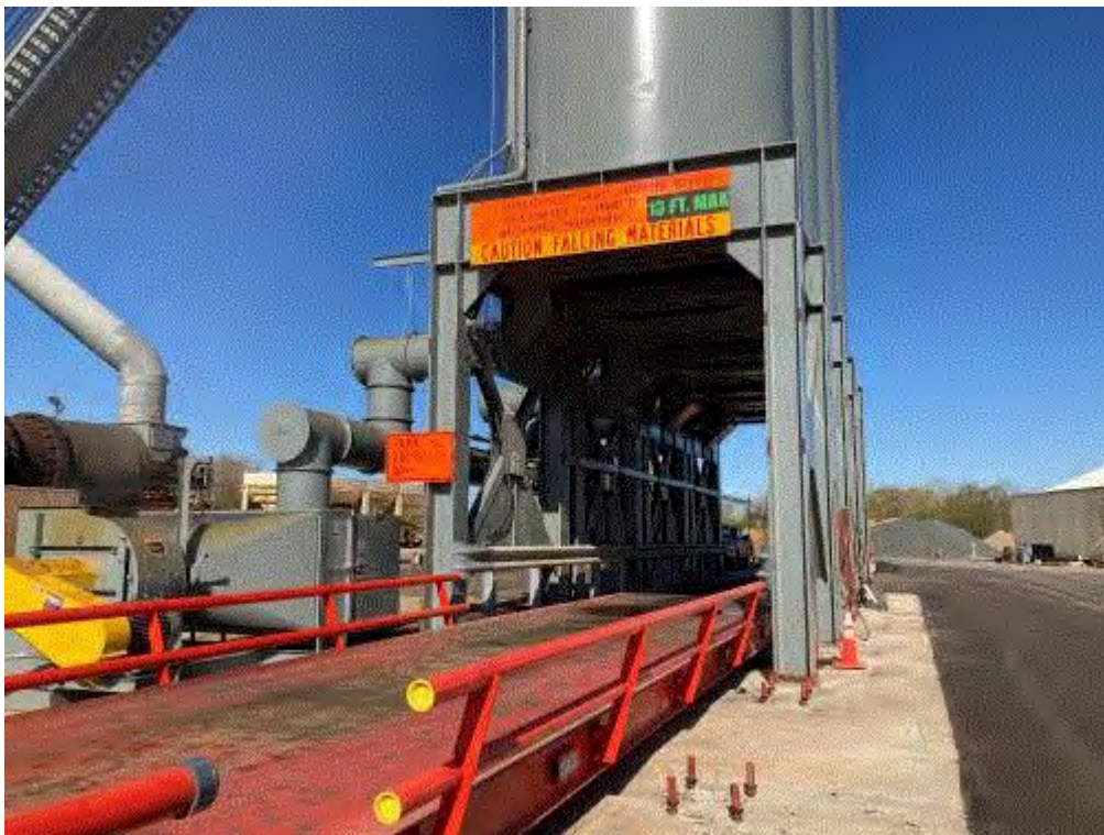
Image 3(Loadout Tunnel) : New loadout tunnel with new control device
