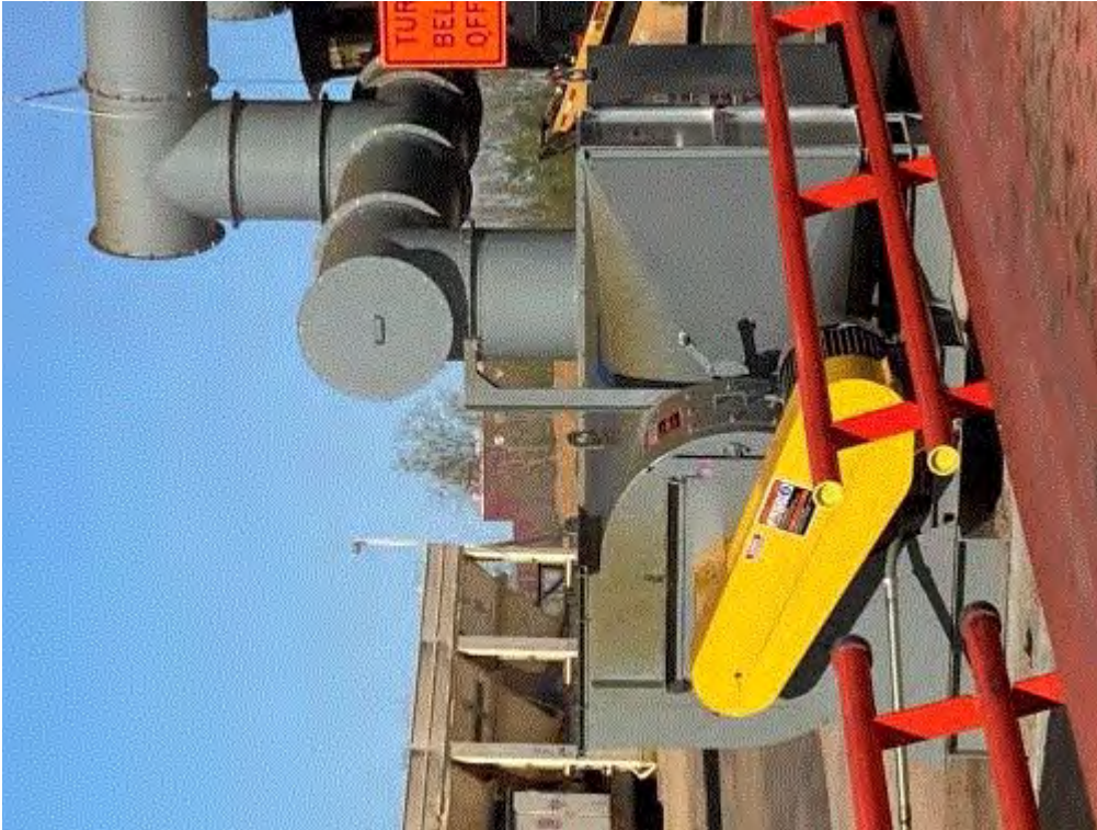
Image 4(Loadout Control) : New control system close-up. No opacity seen from unit during loadout activities.
