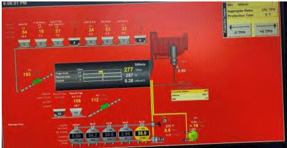
Image 1(Continuous Monitor) : Continuous Monitor screen for product temperature, virgin aggregate feed, RAP aggregate feed, etc.
