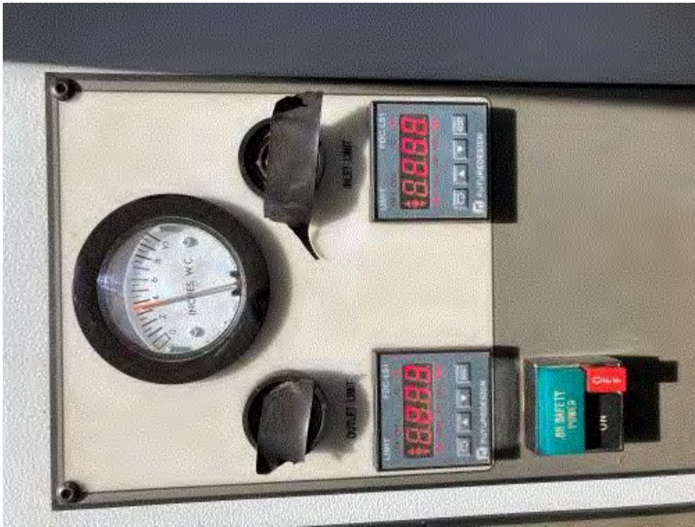
Image 10(Baghouse dP) : Pressure drop monitor for baghouse control. Photo credit: John Berscheid, Rieth-Riley
