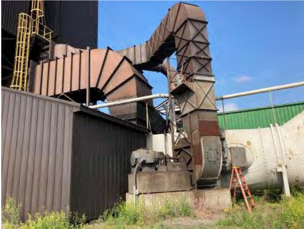
Image 4(EAF Baghouse) : EAG Baghouse elbow area.
