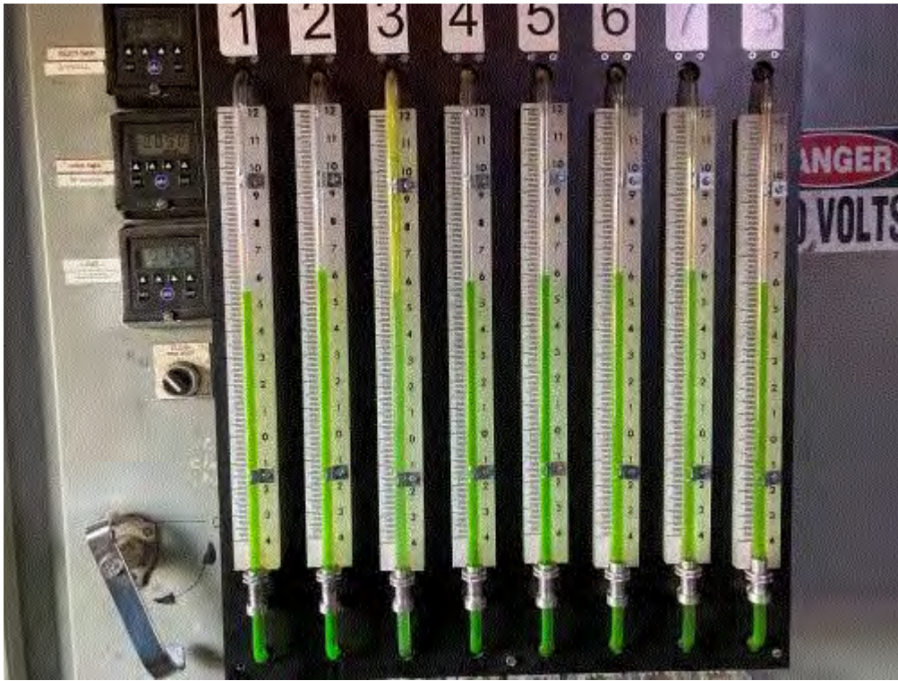
Image 6(EAF Baghouse) : EAG baghouse pressure drop readings for each baghouse section.
