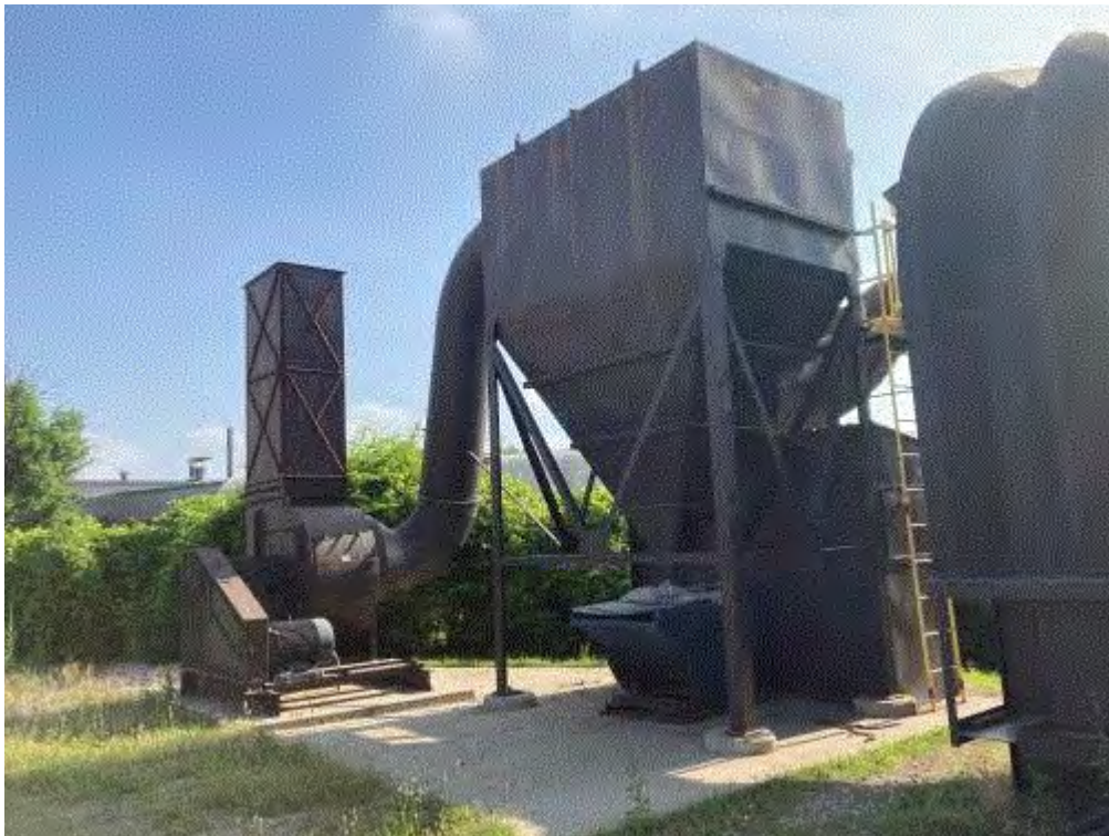
Image 10(Slag baghouse) : North slag building baghouse. (not operating)
