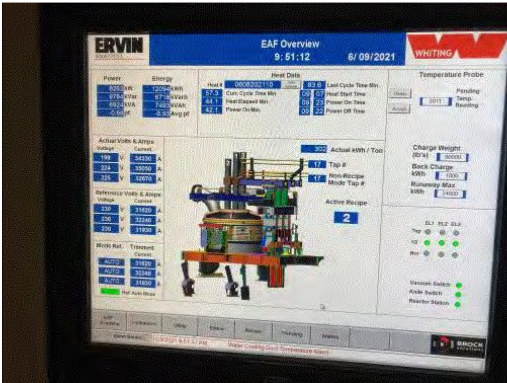
Image 12(EAF Control Room) : EAF Control Room view
