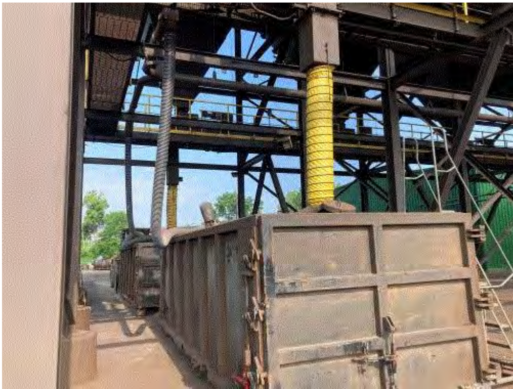
Image 3(EAF Baghouse) : EAG Baghouse boxes where fines are disposed of.
