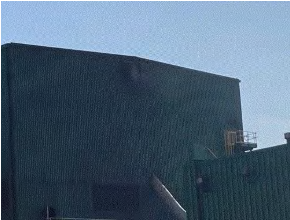
Image 2(South wall-Melt Shop) : South wall-Melt Shop showing roof vent with louver stuck open resulting in opacity.
