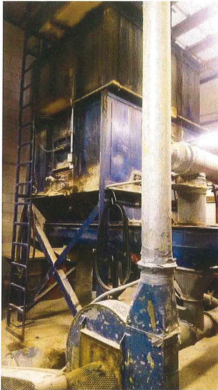
Image 3(R3) : Wood waste handling system cyclone and auger fed delivery system for the boiler.
