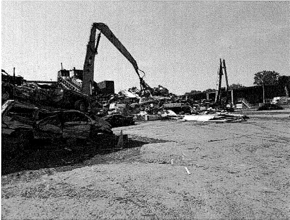
Image 12(Crane) : Crane near shredder
