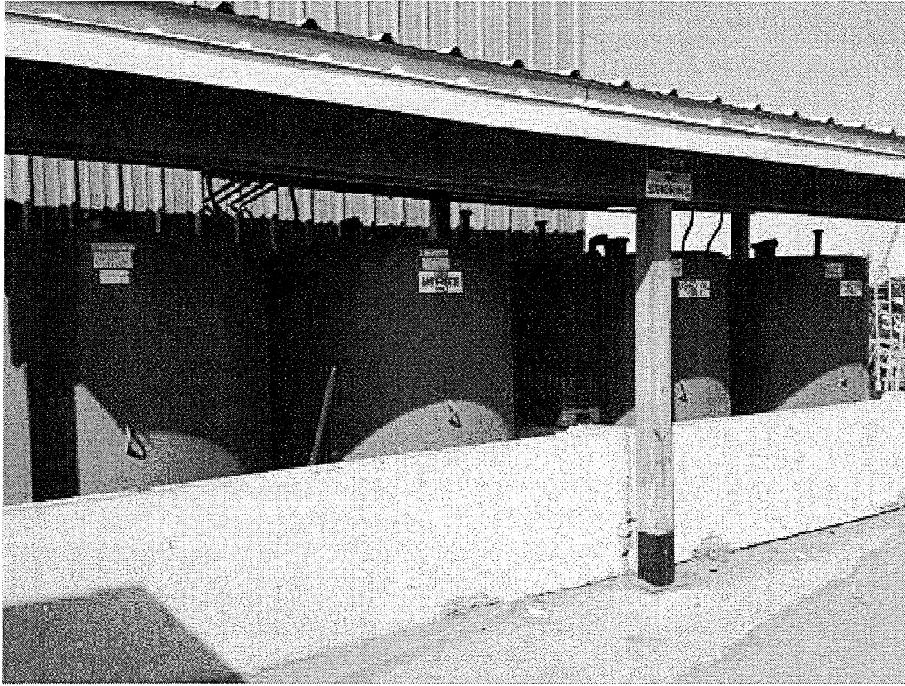
Image 6(storage tanks) : Storage tanks at depollution area
