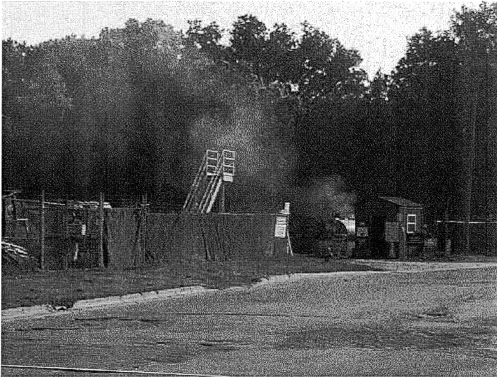
Image 2(Torch Cutting) : Smoke from torch cutting observed when arrived at facility
