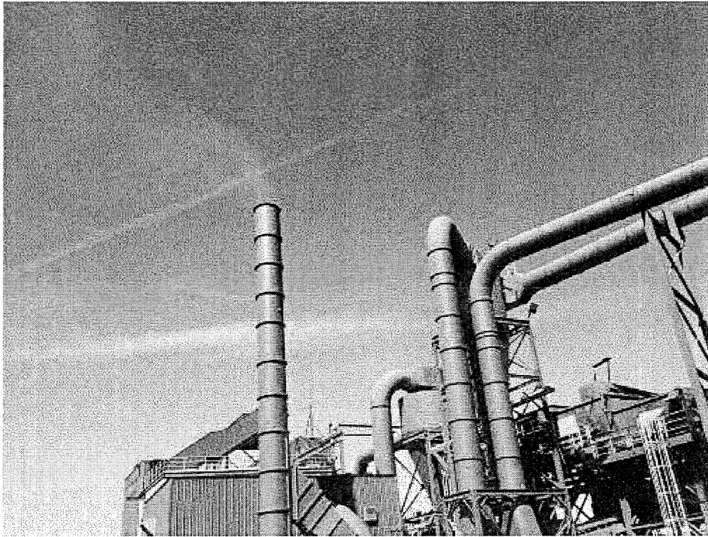
Image 5(Venturi Scrubber) : Venturi scrubber stack showing opacity.
