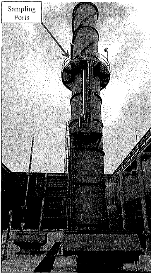
Figure 2-4. SV-MAIN1 Exhaust Stack
