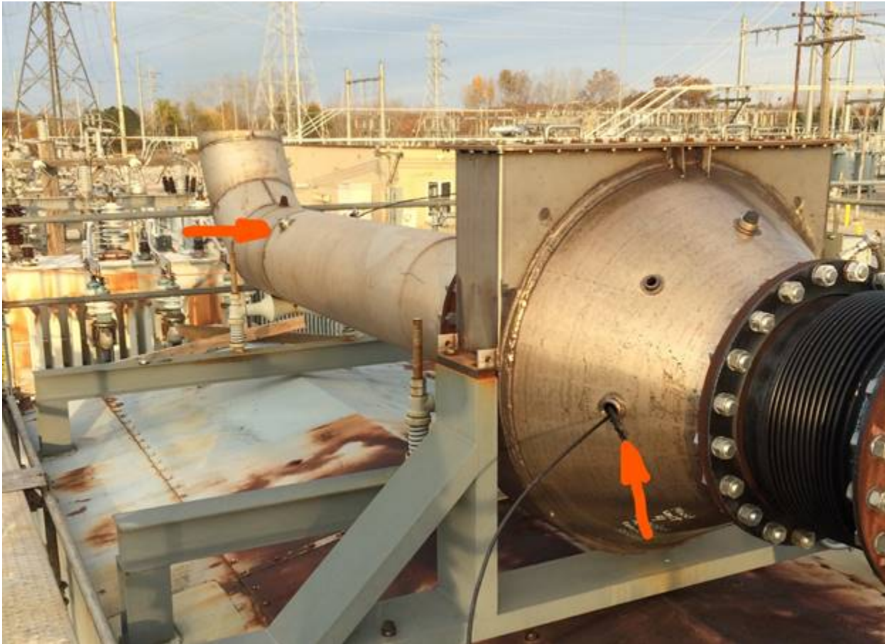
Figure: Catalytic Oxidation system (FGPEAKERS, Design/Equipment Parameters, SC IV.1)
