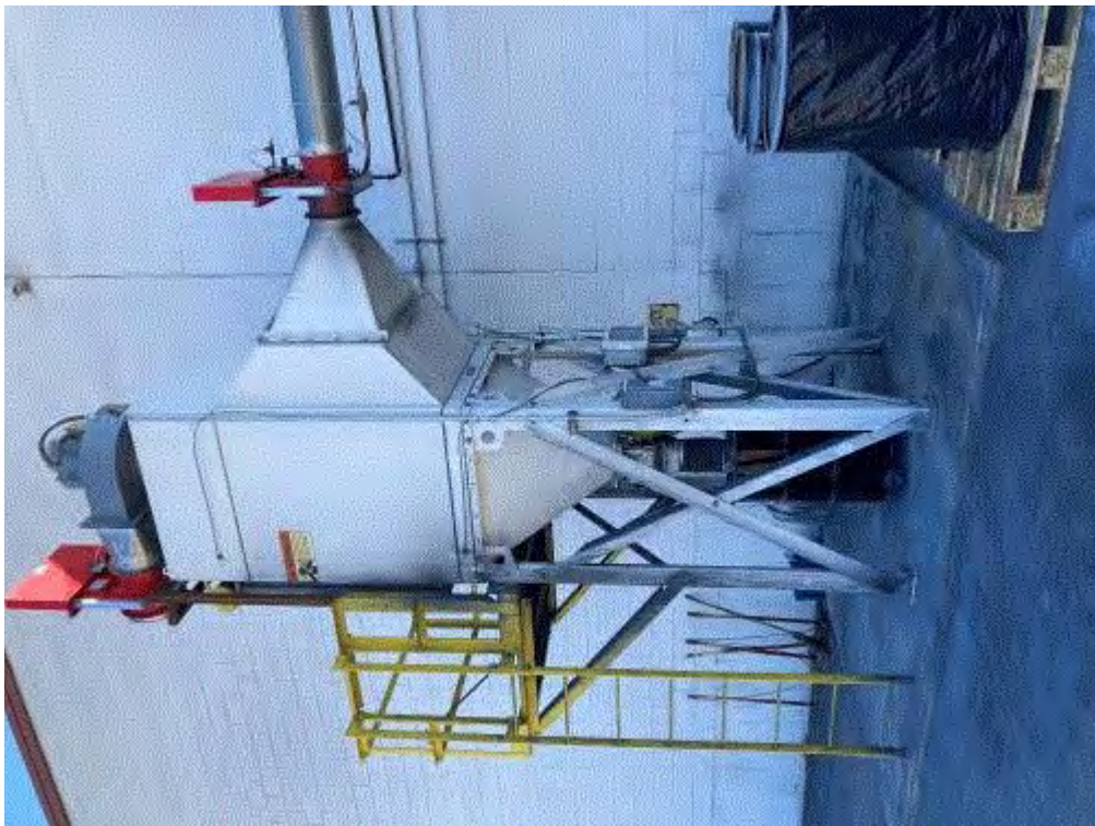
Image 7(Zinc Shot Baghouse) : Note the particulate on the ground, the facility wall, down the sides of the unit,
