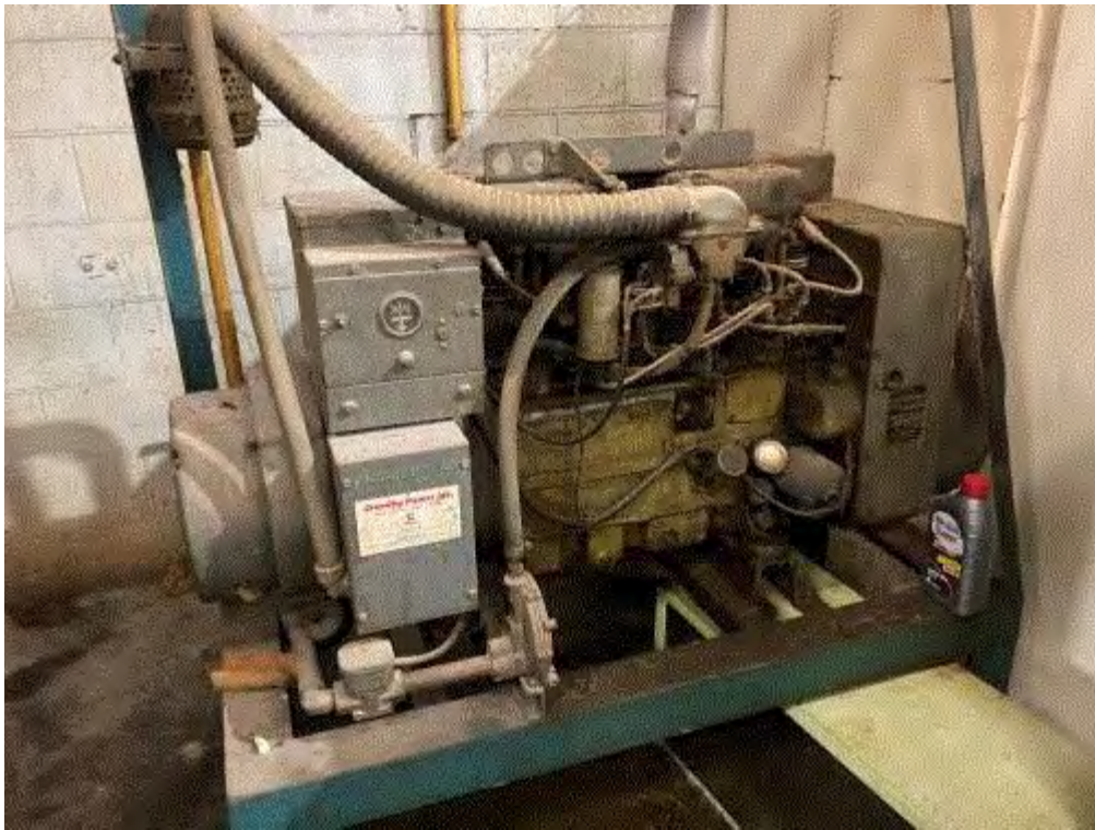
Image 4(Emergency Generator) : Used for IT support & lighting if power went out.
