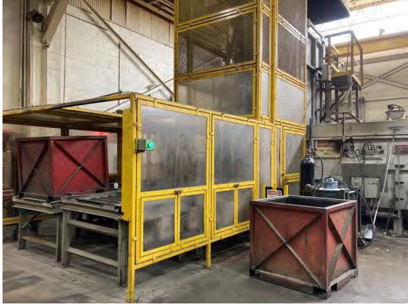
Image 2(Furnace 1106) : Standalone furnace with 1 launder system.
