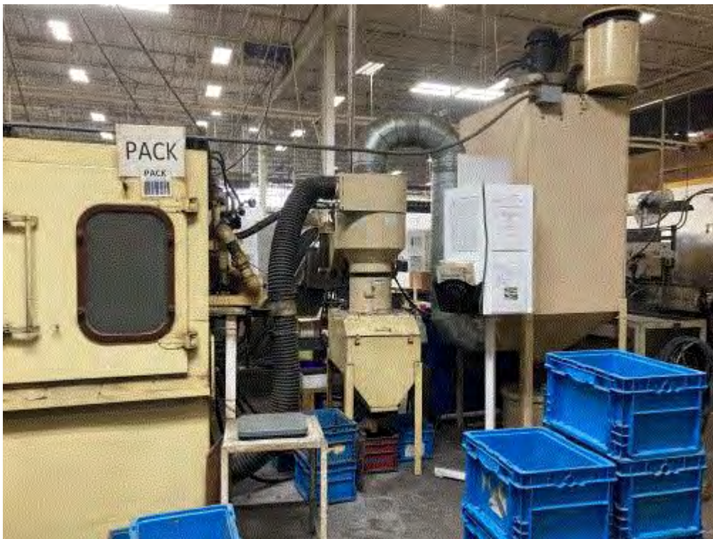
Image 5(Steel Shot) : Steel shot blasting machine venting to in-plant environment post-control
