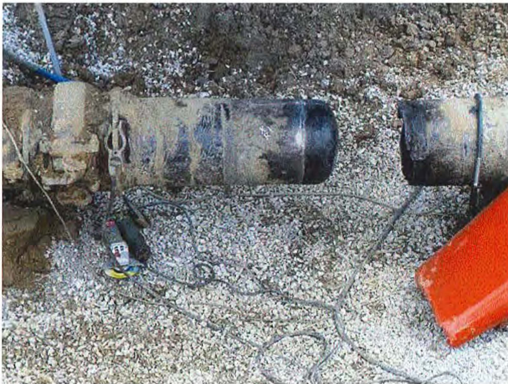
Image 1(001) : Air-gapped line, close up.
