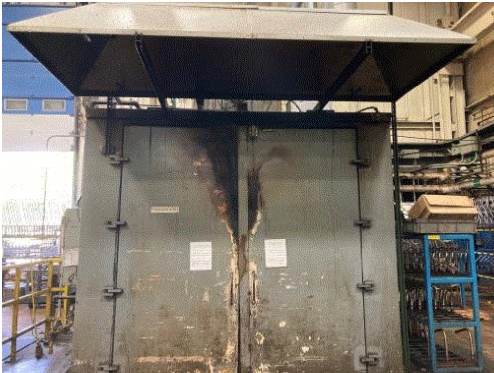
Image 4(Oven doors) : Oven doors with hood above it
