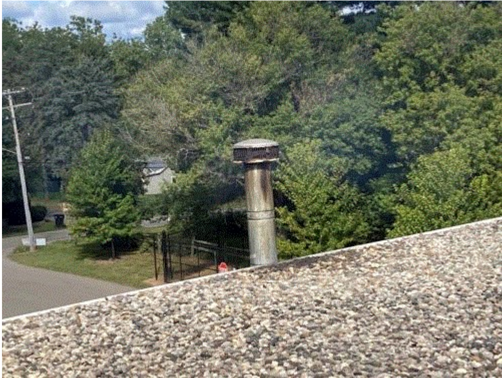
Image 3(Oven stack) : Oven stack showing 10% opacity smoke.
