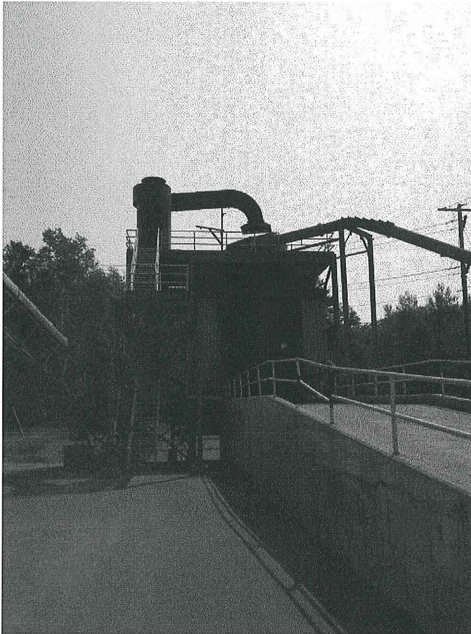
Image 1(LWEC Cyclone) : View of LWEC cyclone fuel receiving hopper, note space between stack and hood. Photo taken 8/27/2015, looking south.
