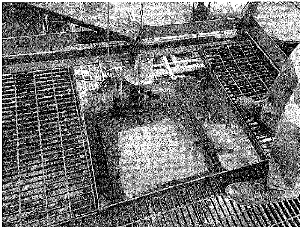
Image 6(Tank Hatch 1) : Asphalt cement tank showing leaking hatch.
