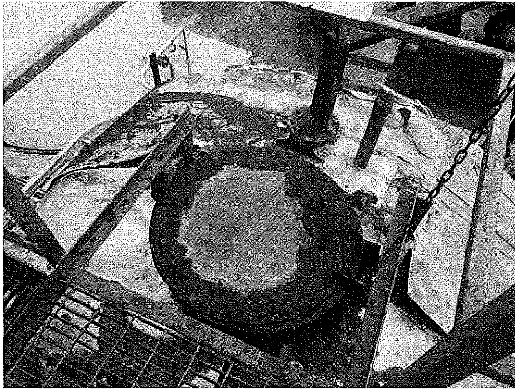
Image 7(Tank 2 Hatch) : Another leaking hatch on an asphalt cement tank.
