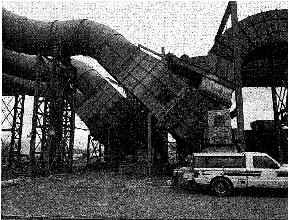
Image 8(Baghouse ducts) : Ducts to Baghouse
