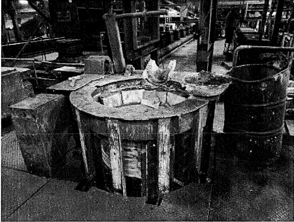
Image 4(broken melt furnace) : broken melt furnace
