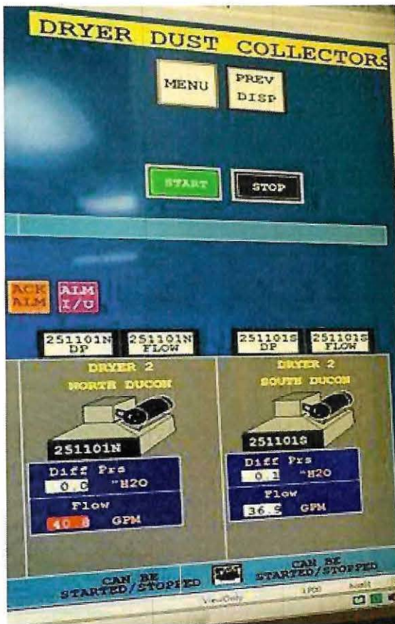
Above are photos of the dryer dust collector/scrubber differential pressure and flow rates recorded during my inspection.
