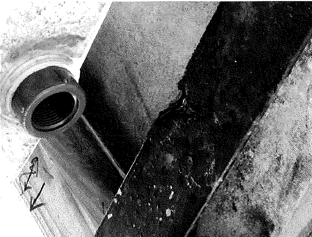
Image 2(Nitric Scrubber) : Metal framework showing acid attack
