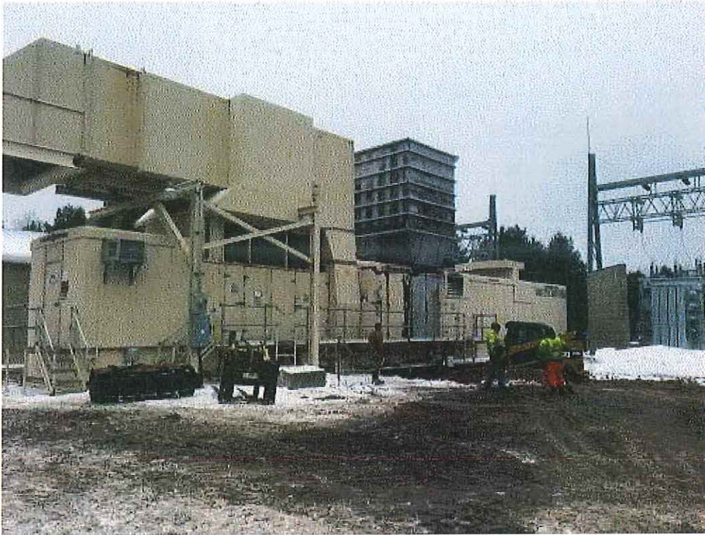
Image 1(Image 1) : Frame 5 genset unit and oil leak remediation
