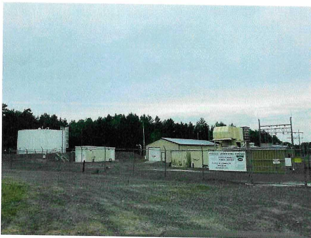
Image 1(UPPCo1) : View of UPPCo Portage Station housing EUGASTURBINE on 8_24_21
