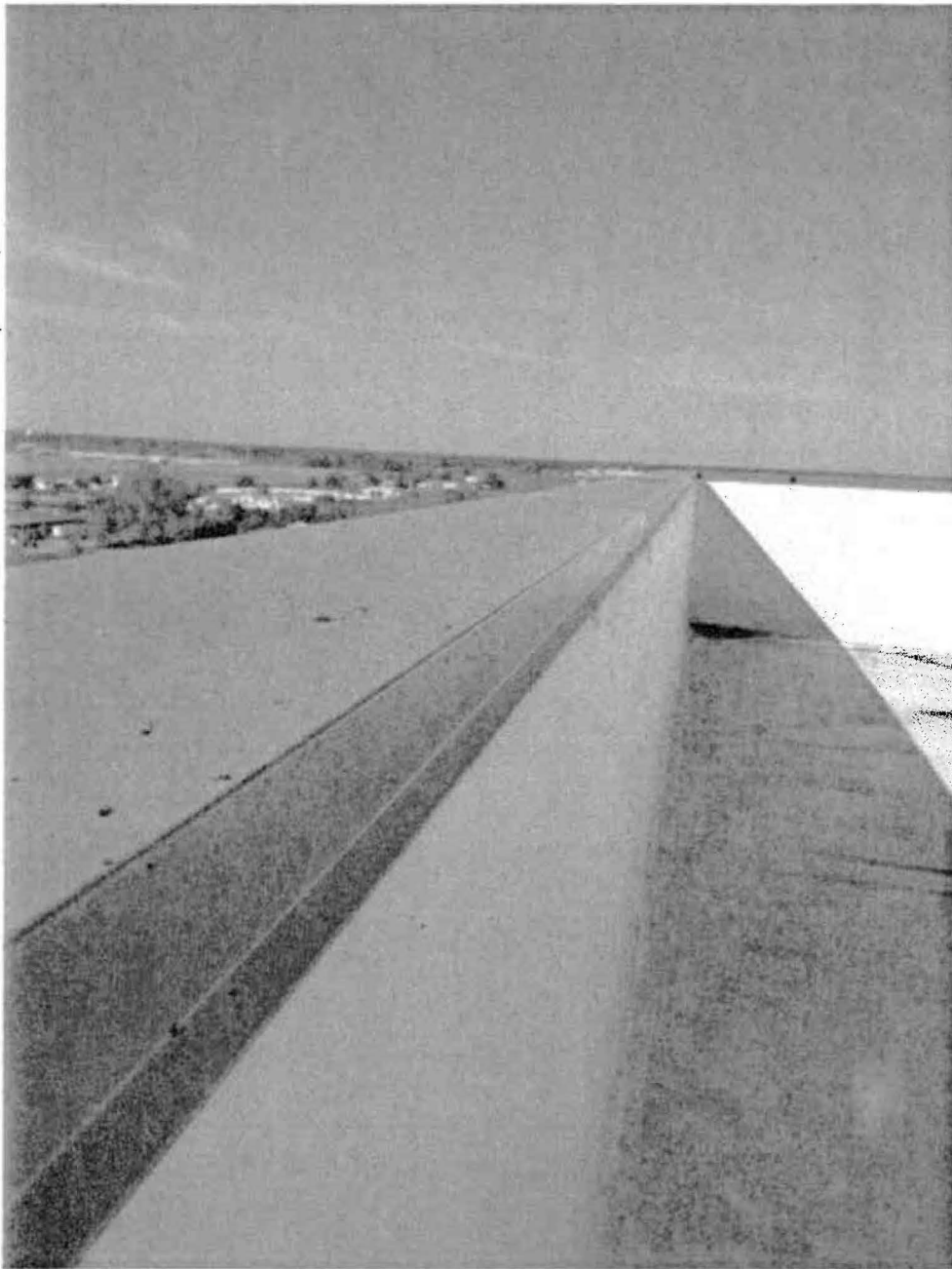
Image 1(Continental roof1) : View of particles on roof ledge at continental. (this ledge is over another lower section of the facility)
