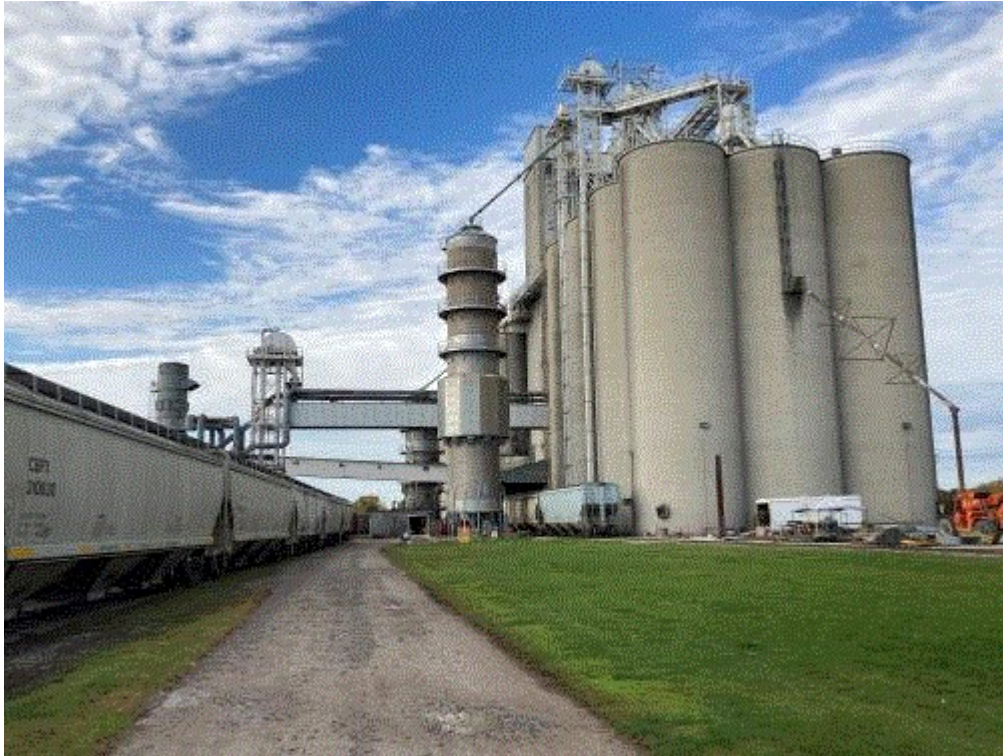
Image 3(Column Dryer) : View of 5,000 bushel per hour Zimmerman column dryer that replaced Berico from PTI #94-80.
