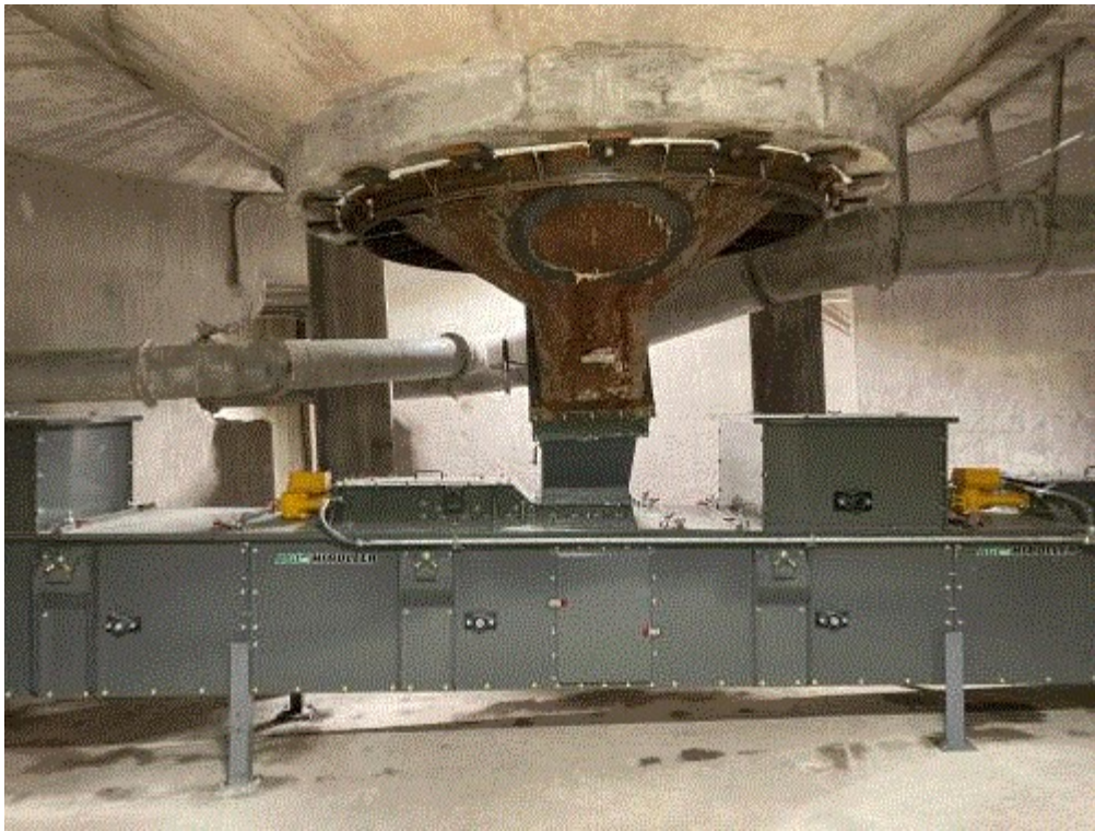
Image 1(Basement Conveyor) : Summer 2023 project enclosing conveyor vents in basement to improve dust handling. Shows how one of the silos connects to the conveyor system.
