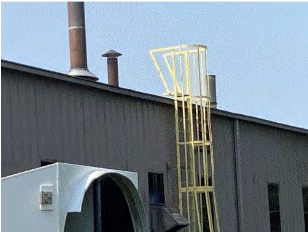
Image 4(4) : Exterior ladder with safety cage not secured to plant roof. Do not climb if not secured.
