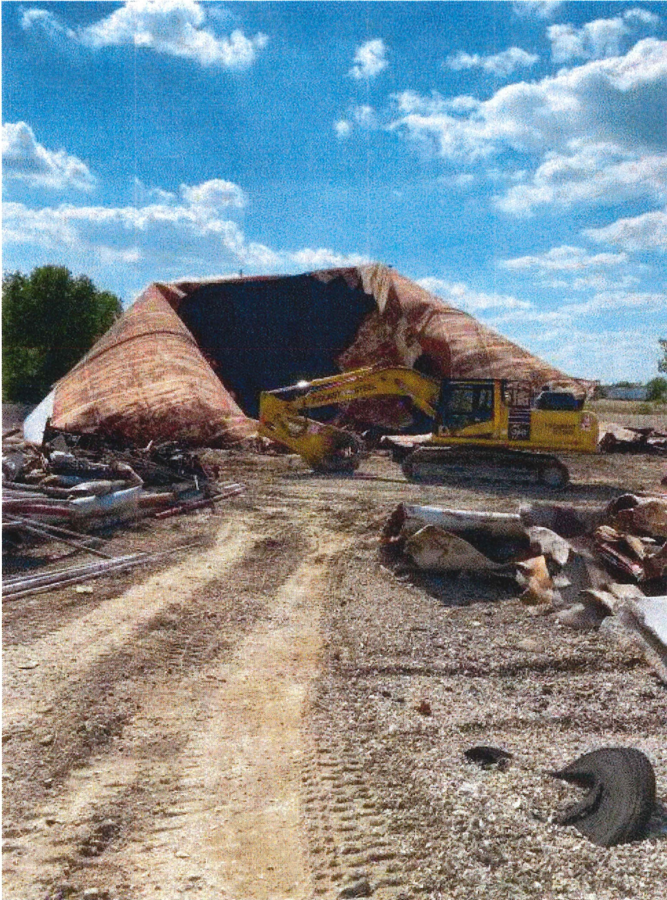
Image 1(Tank Shell) : Image of a tank shell after being dismantled. View from the east side of the property.
