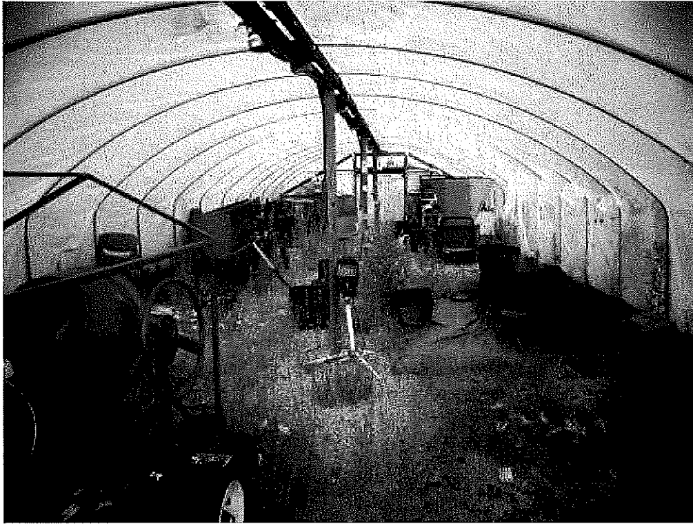
Image 1(Fig. 1.) : Fig. 1. Photo of the green house facility documenting that the oil burner furnace was not installed as planned in PTI No. 26-07,
