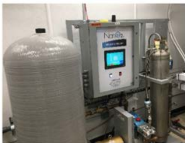
Incoming supply purification tank, control panel, pressurization & saturation tank
