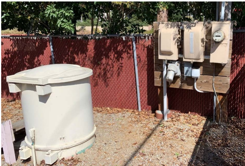
FIGURE 18 CALLED JOAQUIN SEWER PUMP STATION POWER SUPPLY SWITCHGEAR
