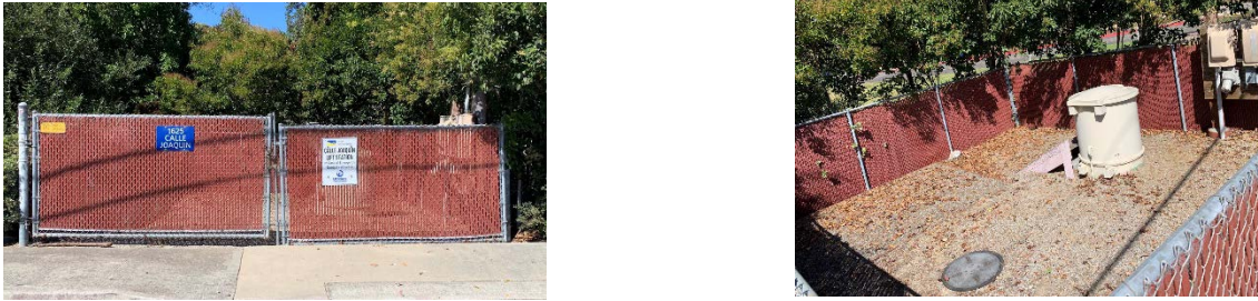
FIGURE 17 CALLE JOAQUIN PUMP STATION
