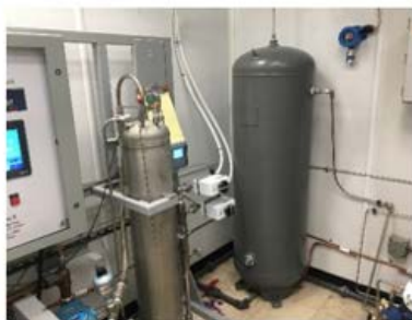
Pressurization & saturation tank, incoming supply holding tank
