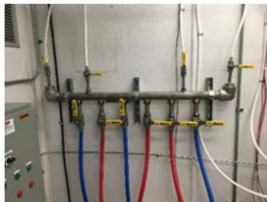
Outbound emulsion manifold
