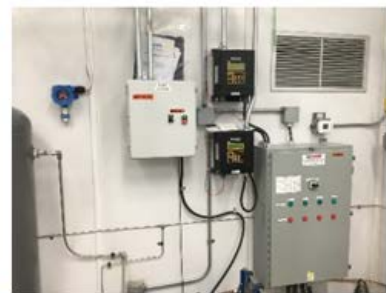
Power supply control, 480 volts
