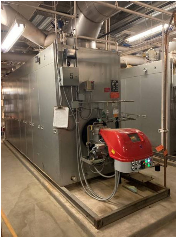
Image 1: Boiler 5 hot water heating boiler
