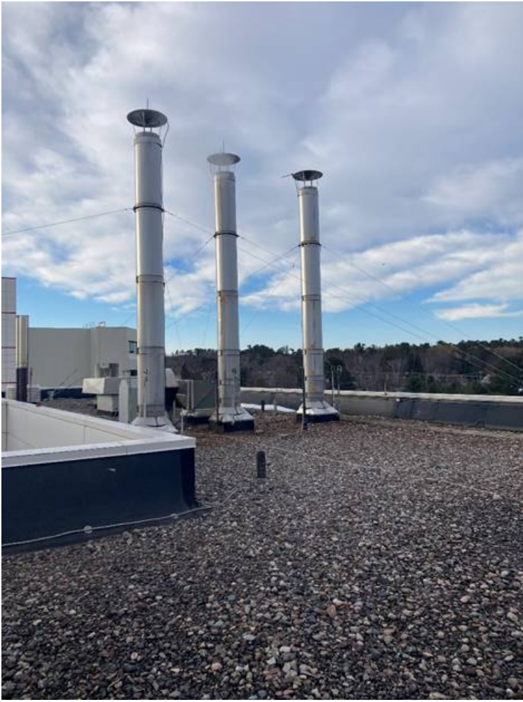
Image 3: Heating Boiler Stacks
