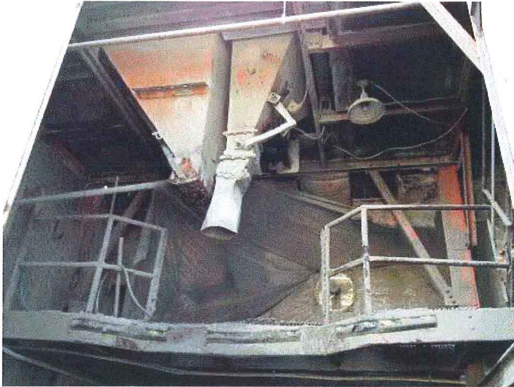
Image 3(MC3) : Load-out bins and chute
