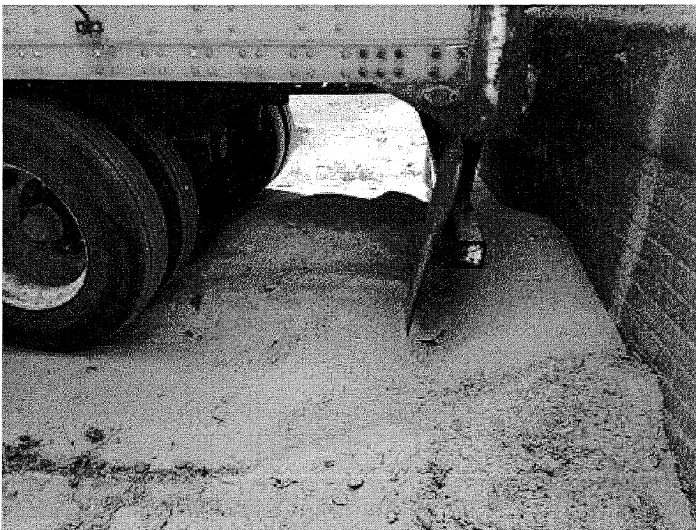
Image 9(Dust on ground) : Dust on ground.
