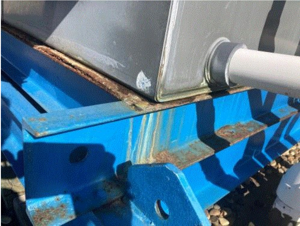
Image 3(Chrome plate) : Liquid leak from stage 1 of scrubber, causing deterioration of structural support.
