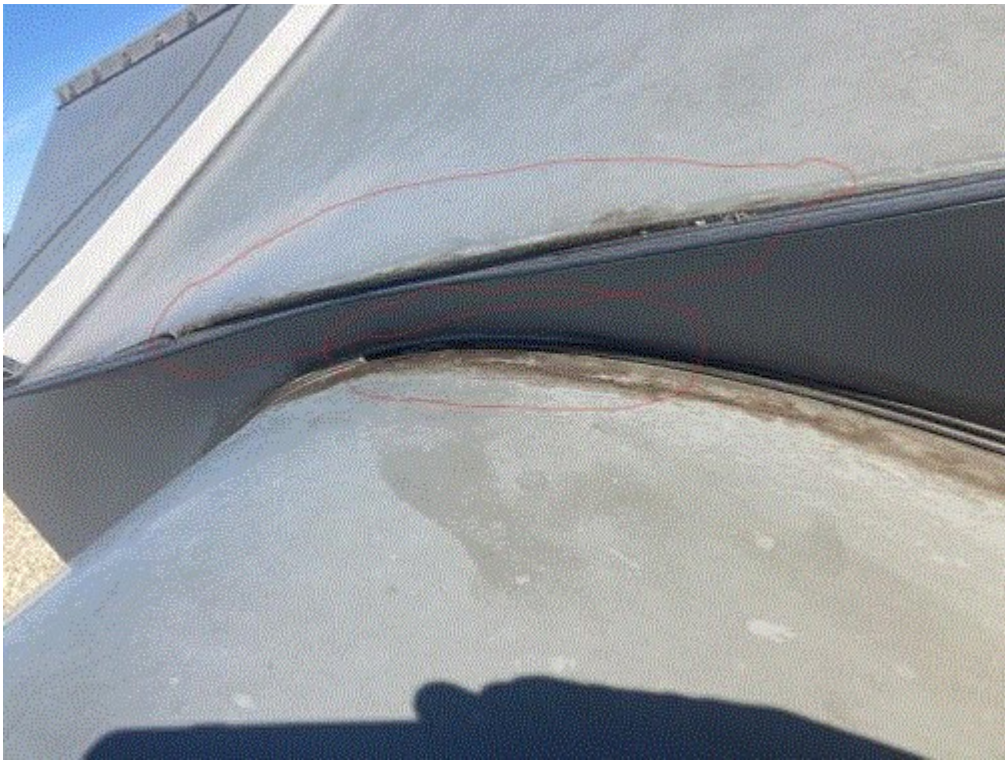
Image 1(Chrome plate) : Areas where two seams have separated, allowing for air infiltration on the inlet side of the hexavalent chrome plating scrubber.
