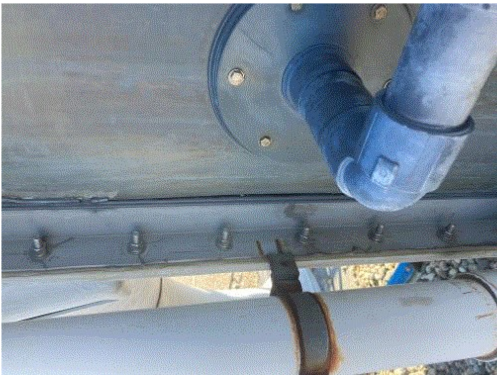
Image 4(Chrome etch) : Seam separation at stage 1 of chrome etch scrubber allowing for air infiltration.
