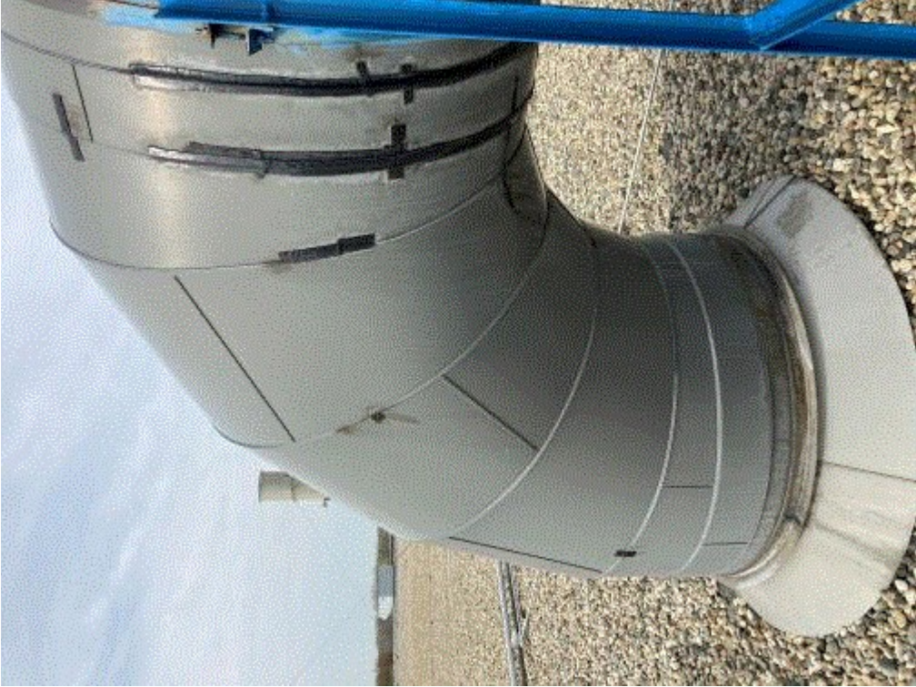
Image 5(EUPN-12) : Chrome plate scrubber inlet ductwork.
