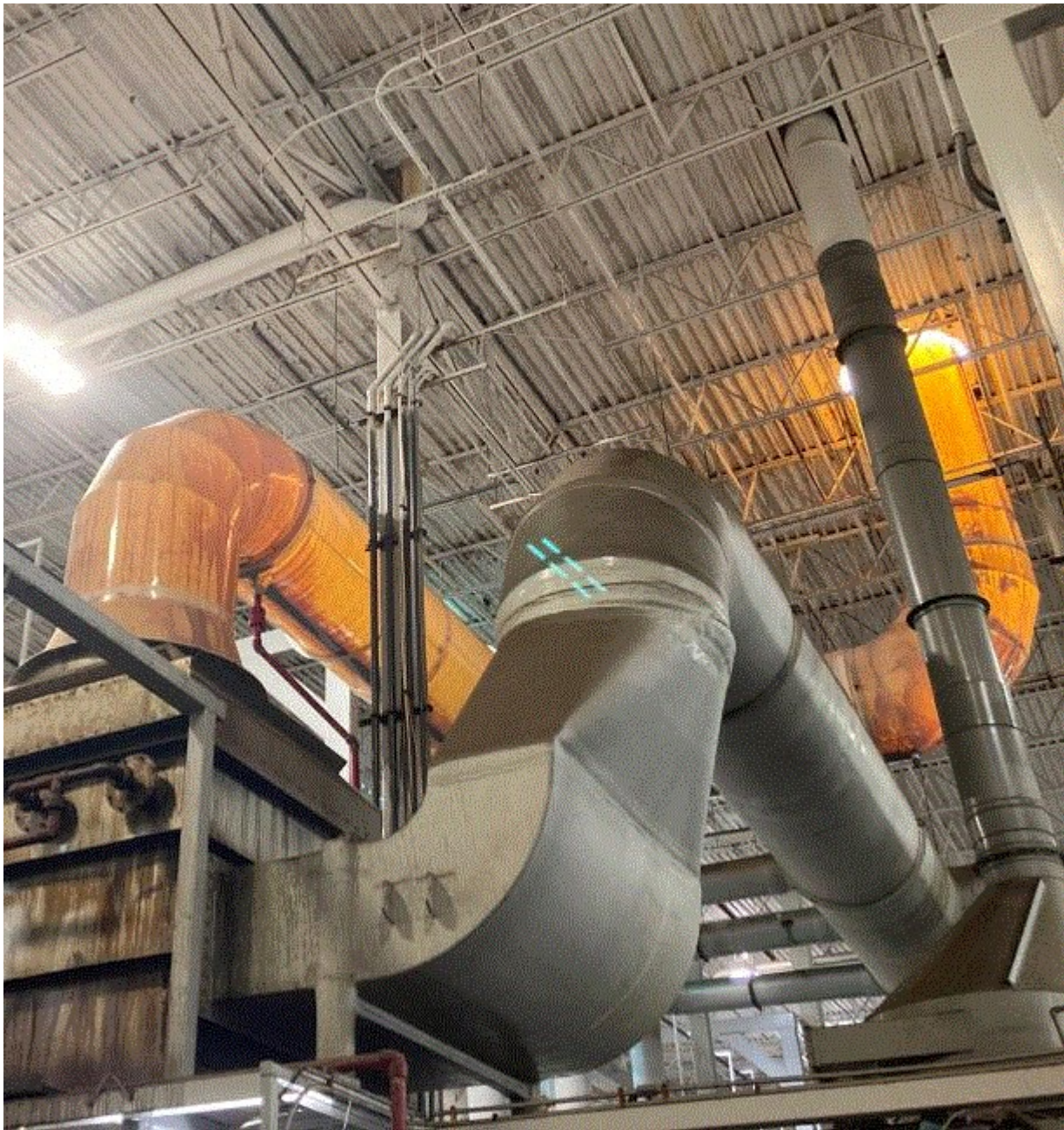
Image 7(EUPN-10) : Photo provided by Lacks of the Kynar ductwork from the evaporator to the roof and scrubber inlet.
