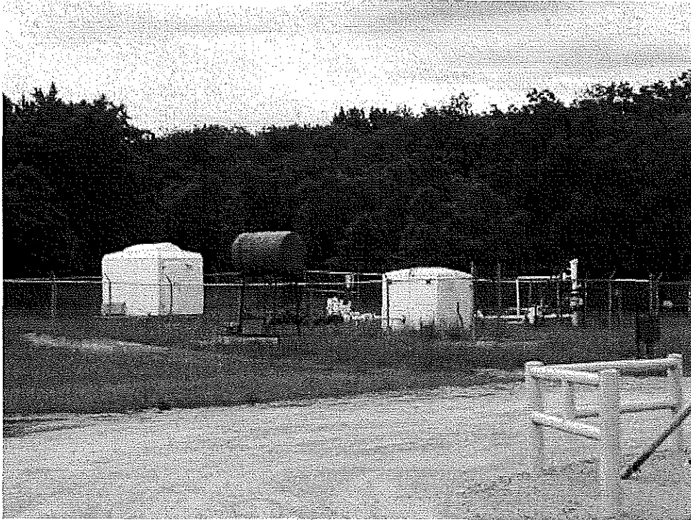
Image 1(DTE Metering) : View of DTE metering station located at the SE end of the facility. Note green tank has been relocated there from the fresh water injection station located immediately west of the metering station.
