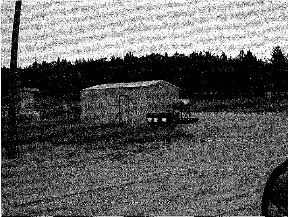
Image 10(water injection) : view from SW of active fresh water injection station. Facility personnel reports that water is not transported offsite, but is reinjected into injection well onsite.
