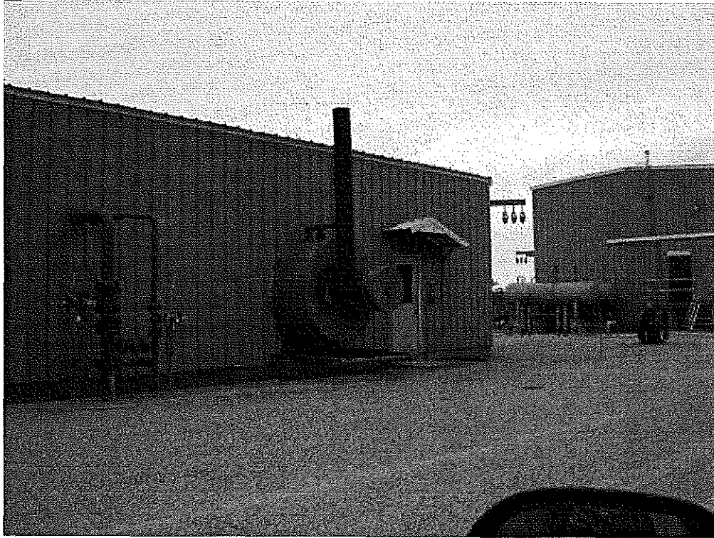
Image 4(in-line heater) : View of inline heater (operating) and associated stack located at the NW end of the dehy building.
