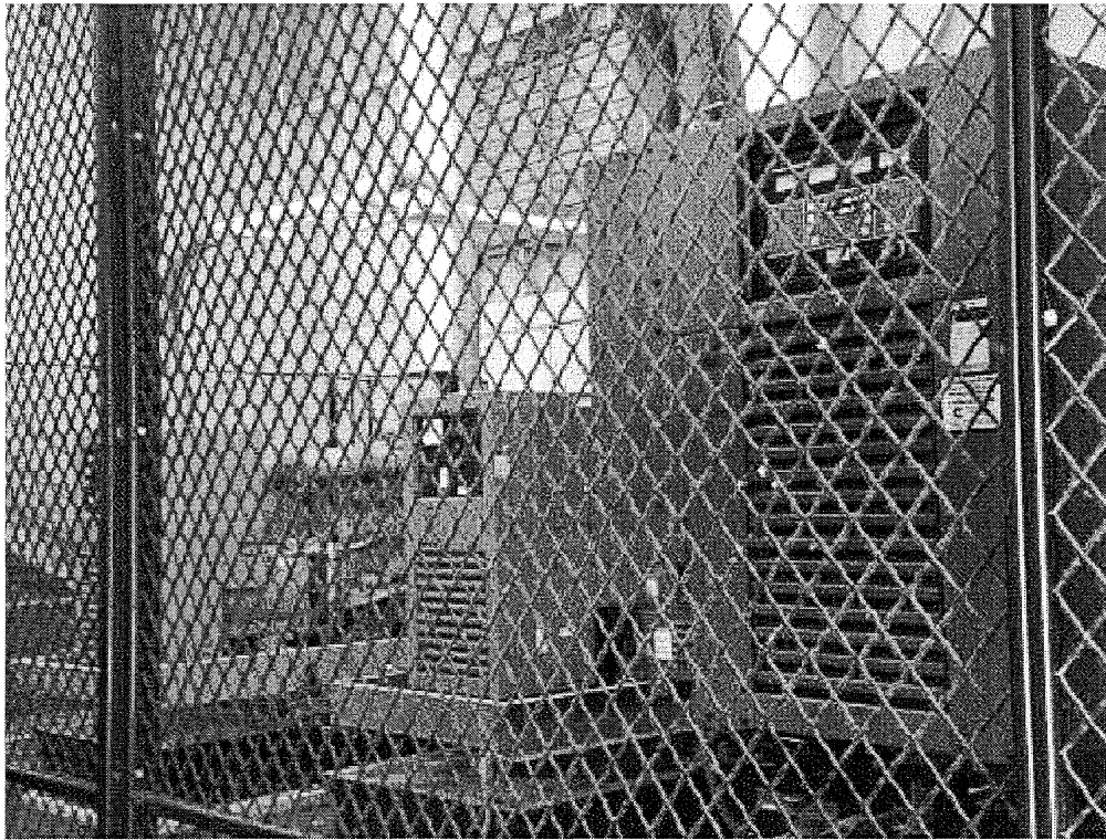
Image 2(Emergency generators) : Some of the emergency generators
