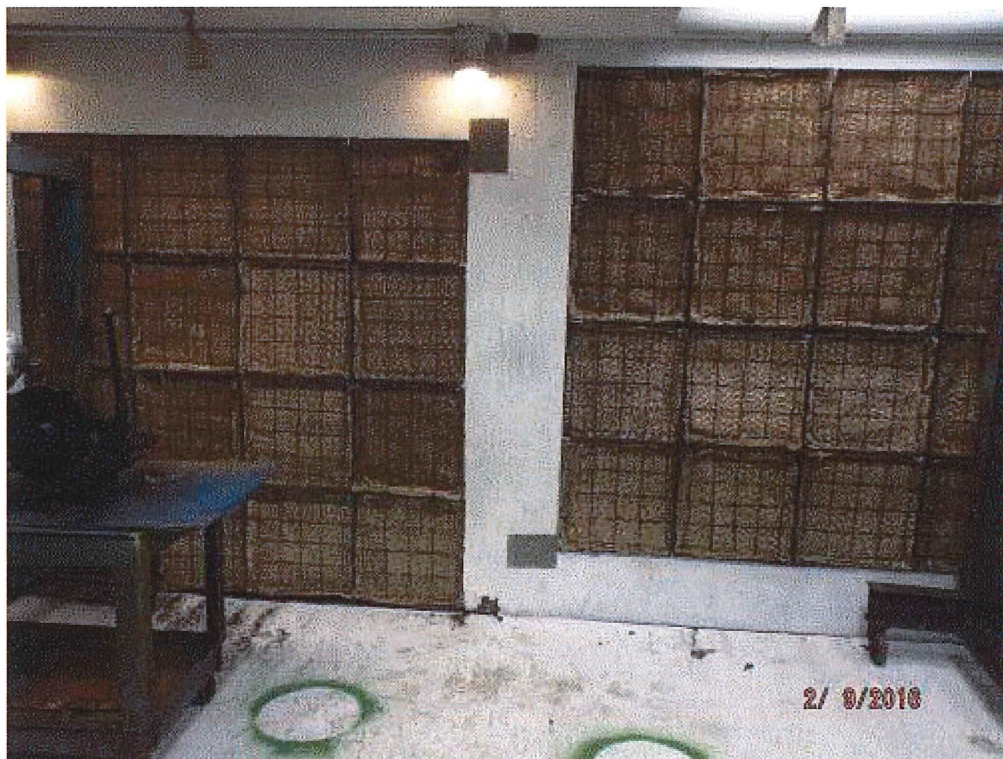
Image 1(DSCF4342.JPG) : Photo provided by H&P Technologies on February 9, 2016. Note the two dark rectangles located between the filter banks. These rectangles are patched areas to prevent particulates bypassing the filters.
