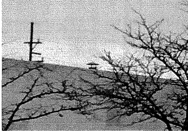
Image 1(Photo 1) : Burnoff oven rain cap.
