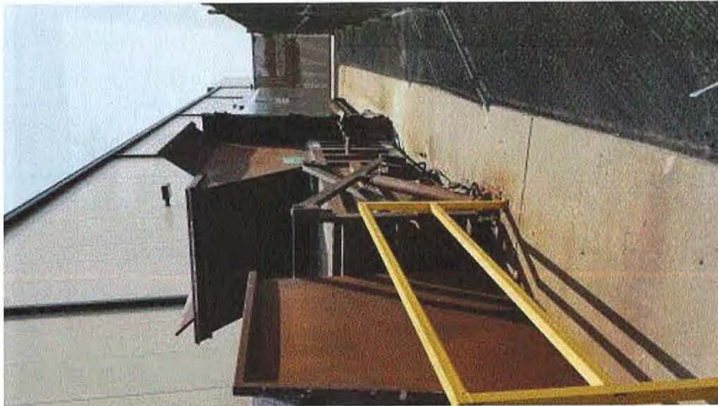
Image 6(Garbage Compactor) : Garbage compactor where bondo dust was seen on the ground. Remedy has been proposed. See inspection report.
