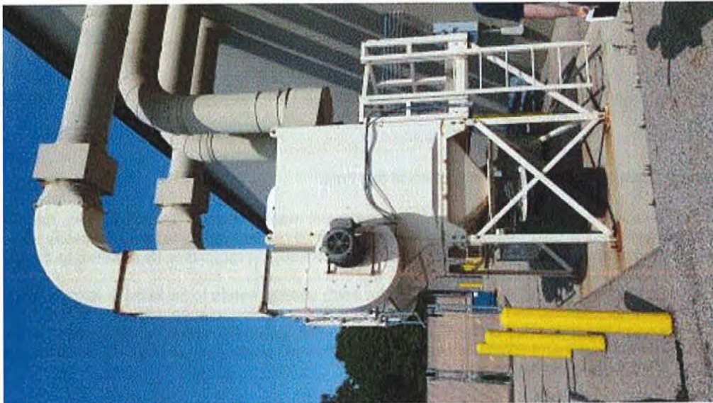
Image 2(Dust Collector) : Dust collector that services the metal grinding, metal cutting, and sanding/buffing stations.
