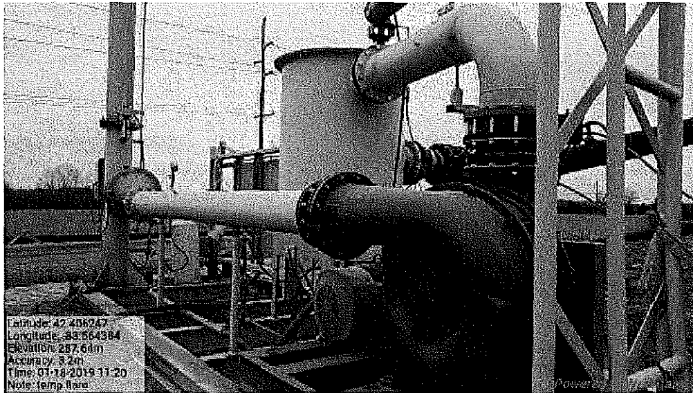
Image 7(Temp Flare) : Temporary Flare.
