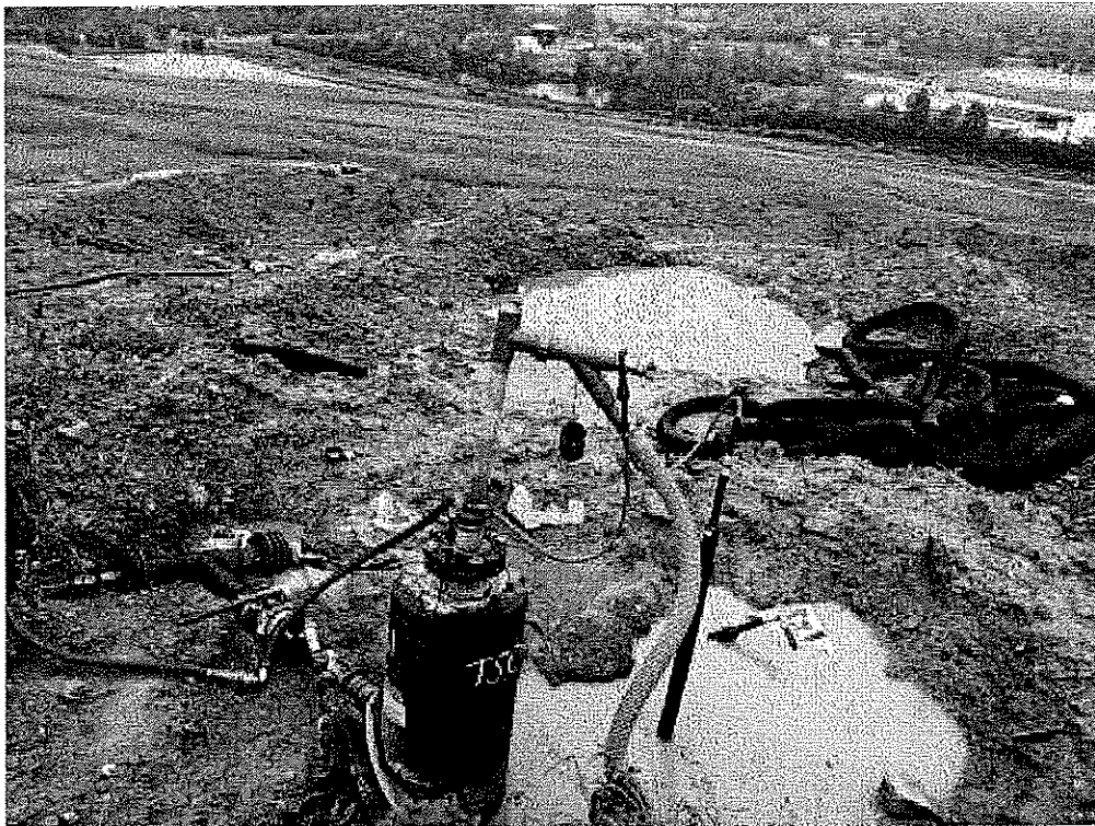
Image 5(TS-01) : TS-01 sump ponds.
