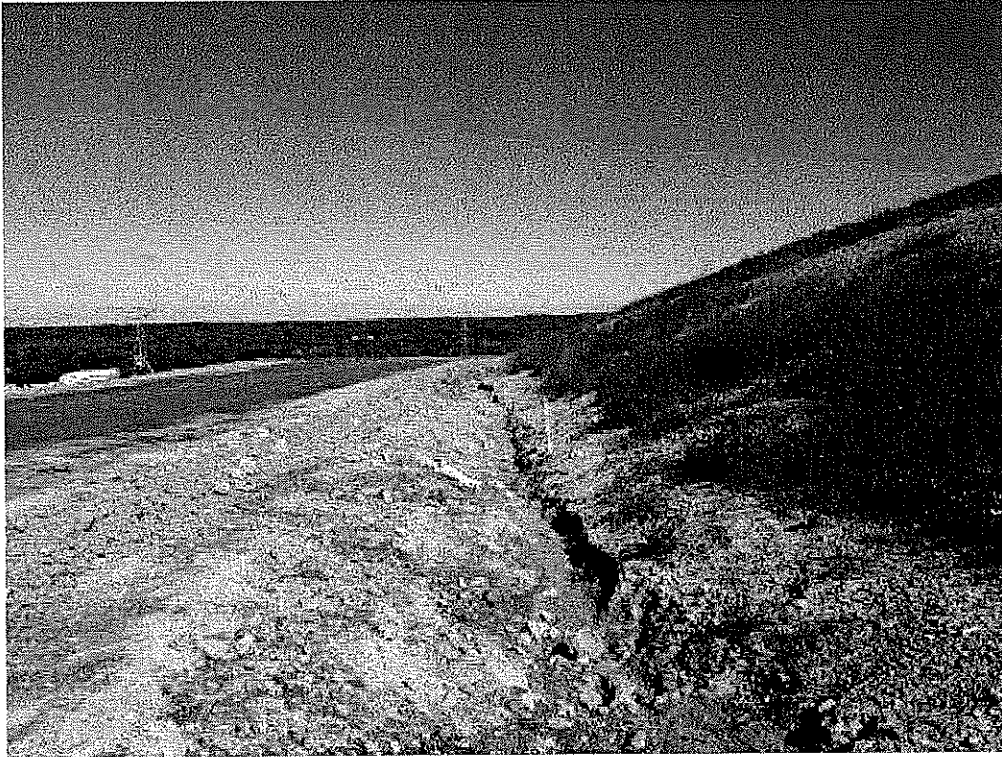
Image 4(West haul road ditch) : West haul road ditch were horizontal well is going in marked with yellow pole.
