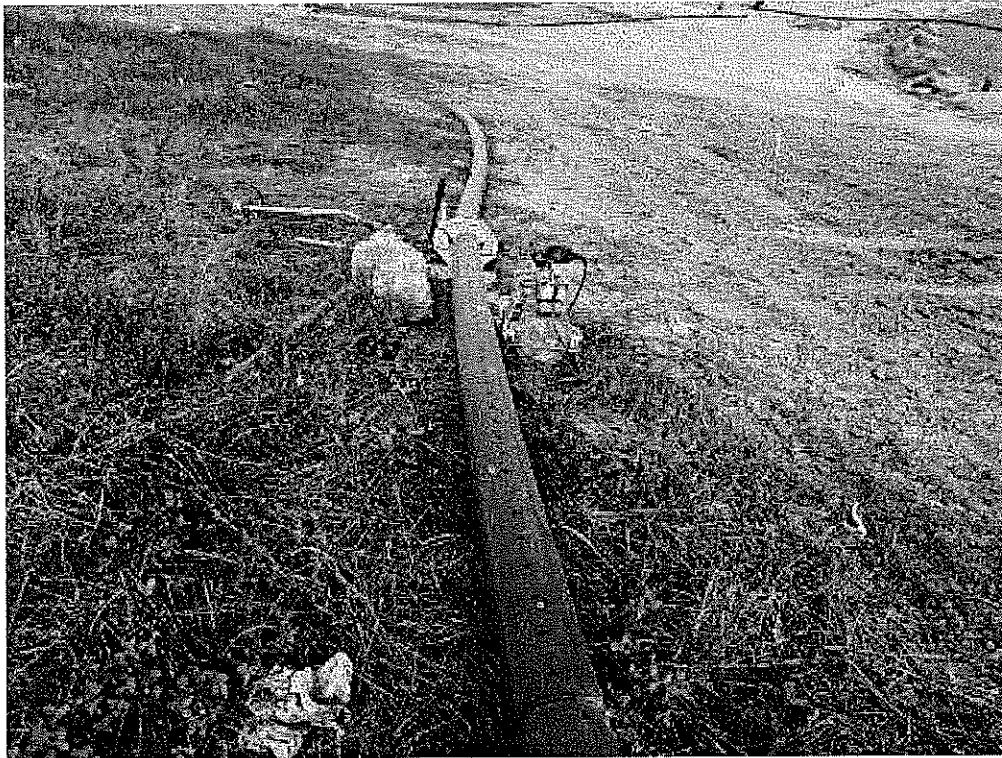
Image 3(Well pipe) : Perforated pipe to be used for new horizontal well on North side.
